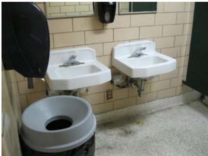
Non-ADA Compliant Wall Hung Lavatories
