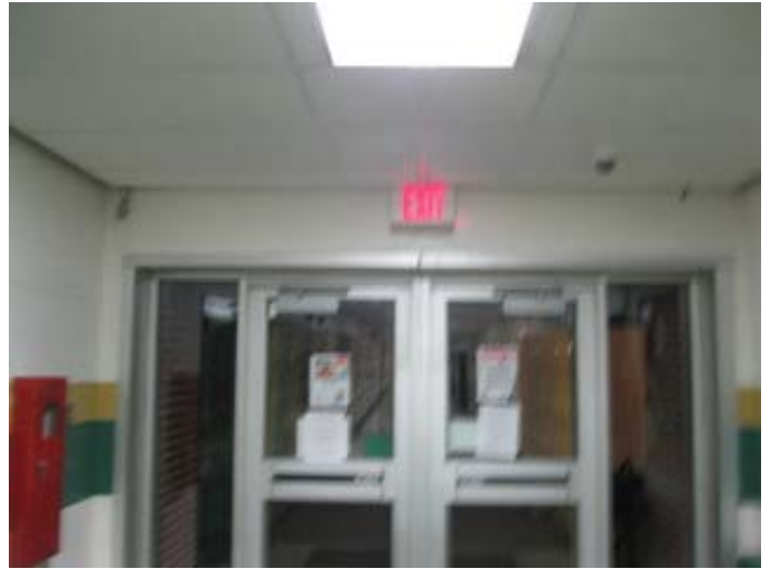
Non-Compliant Exit Sign
