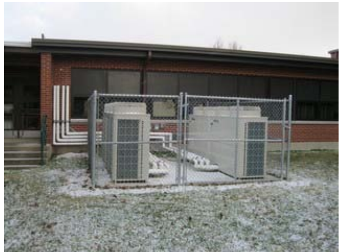
Mitsubishi Electric Fired VRF Heat Pump Condensers
