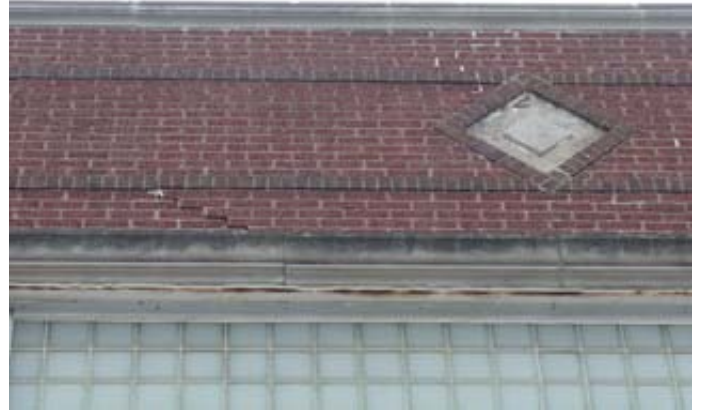
Masonry Repair Needed in 1918 Original Construction
