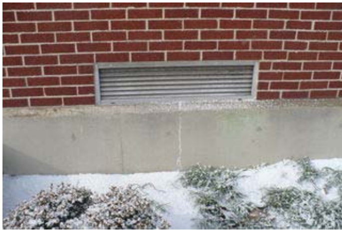
Typical Foundation Crack in the 1951 Addition
