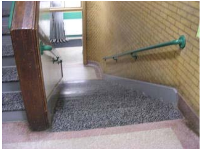
Typical Non-Compliant Stairs/Hand Rails
