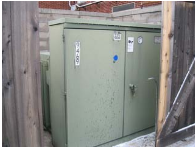
Pad Mounted Transformer
