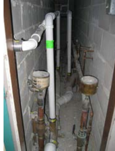
Sanitary Waste Piping
