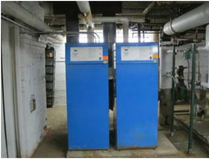
Patterson-Kelley Thermific Natural Gas Fired Heated Water Boilers
