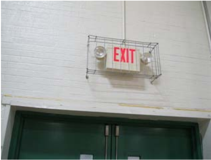
Non-Compliant Exit Sign and Emergency Egress Light Fixture
