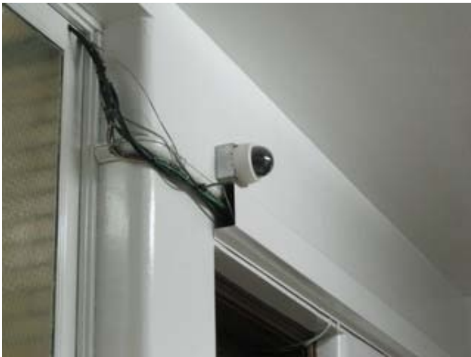
Security System CCTV Camera
