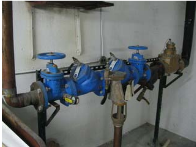
Incoming Domestic Water Service Line
