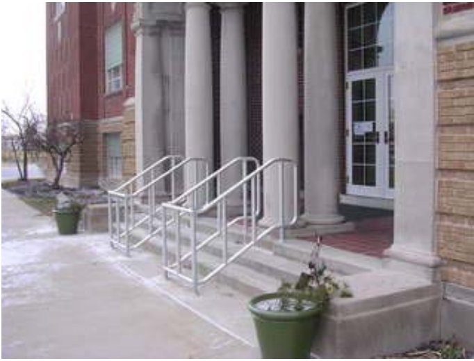
Non-Compliant Main Entry Stairs
