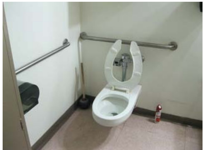
ADA Compliant Wall Hung Flush Valve Toilet
