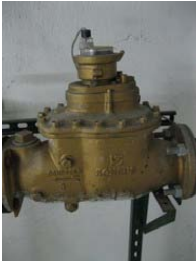
Incoming Domestic Water Service Meter
