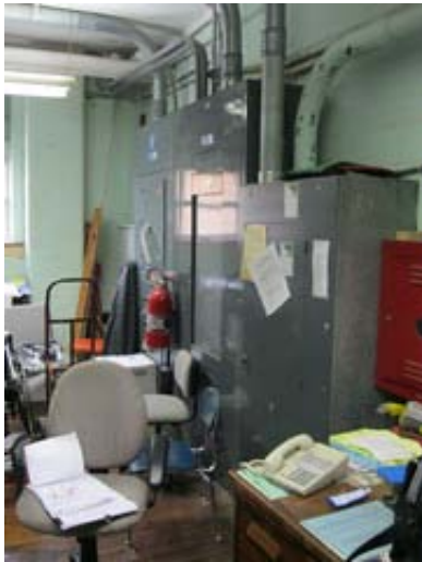
Main Electrical Distribution Panel
