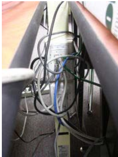
Typical Data Outlets at Classrooms
