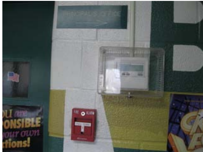
Fire Alarm System Manual Pull Station
