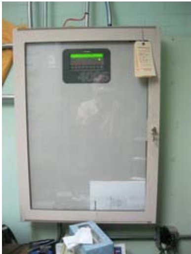
Fire Alarm Control Panel
