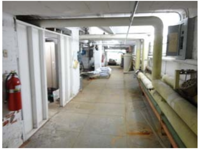
Asbestos Pipe Insulation
