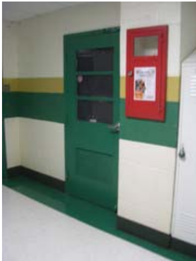
Typical Fire Extinguisher Cabinets
