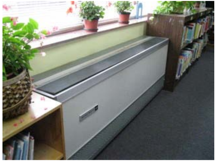
Heating Water Unit Ventilator
