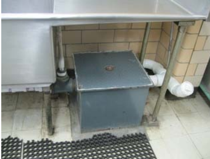
Kitchen Grease Trap Interceptor
