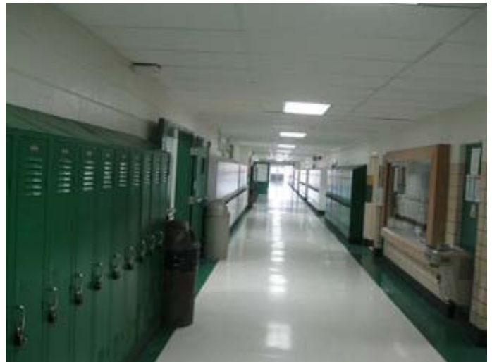
Corridor T-8 2x4 Lay-in Direct Fluorescent Light Fixtures
