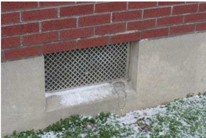
Cracks in the Concrete Foundation Base
