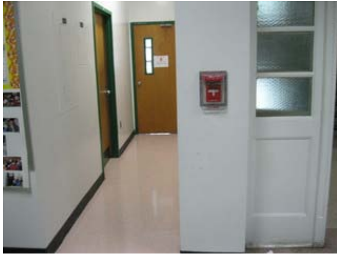
Fire Alarm System Manual Pull Station
