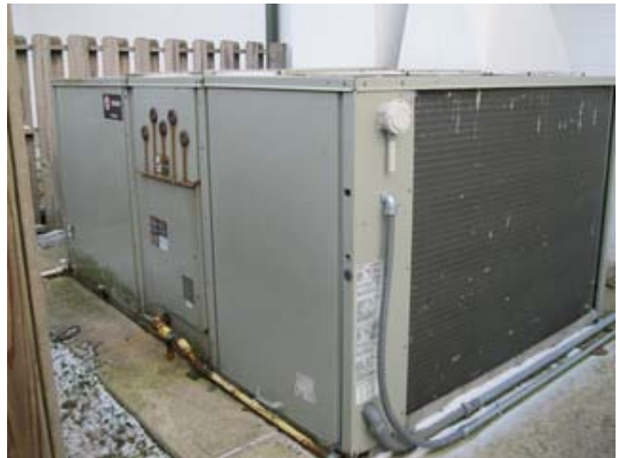
Trane HVAC Unit
