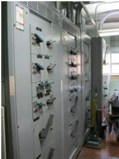
Main Electrical Distribution Panel
