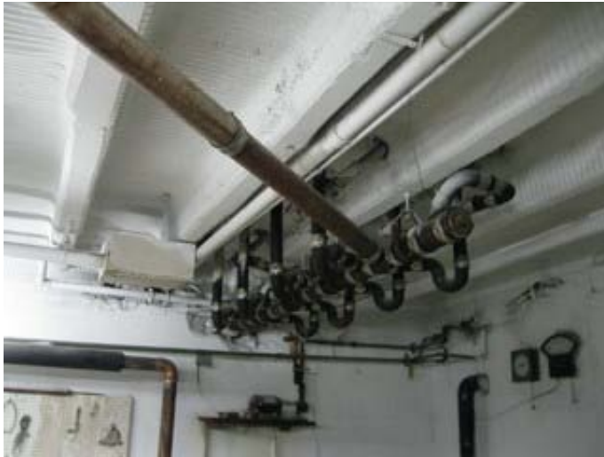
Sanitary Waste Lines
