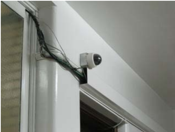
Security System CCTV Camera
