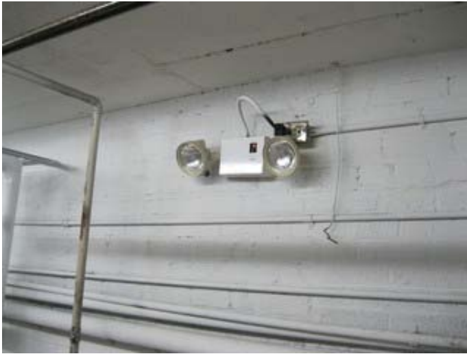
Non-Compliant Emergency Egress Light Fixture
