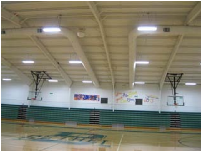
Gymnasium T-8 2x4 Suspended Fluorescent Light Fixtures
