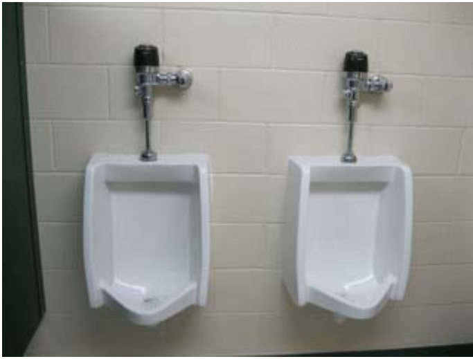
Non-ADA Compliant Wall Hung Infra-red Urinals
