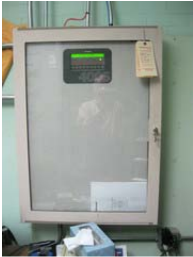
Fire Alarm System Control Panel
