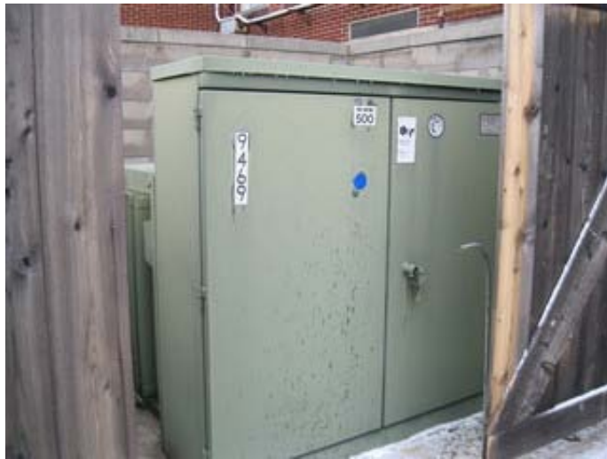
Pad Mounted Transformer
