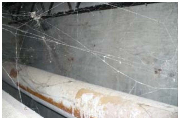
Asbestos Pipe Insulation
