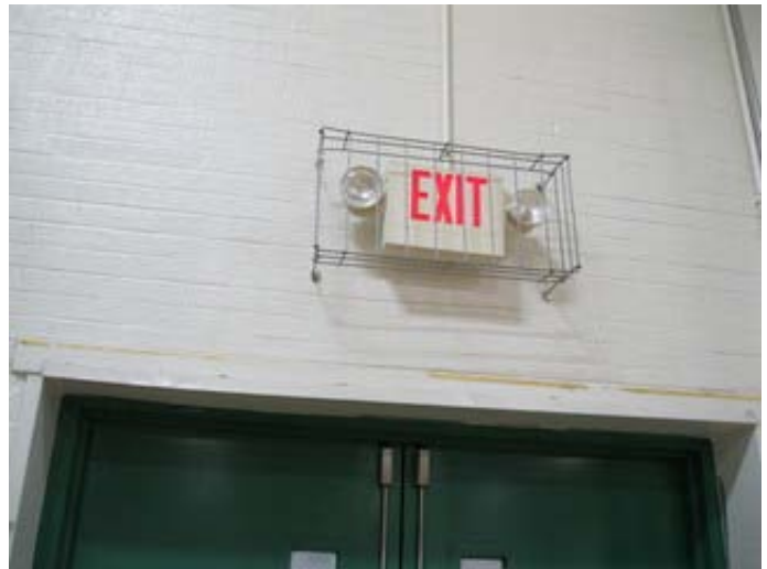
Typical Exit Lighting Signage
