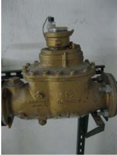
Incoming Domestic Water Service Meter
