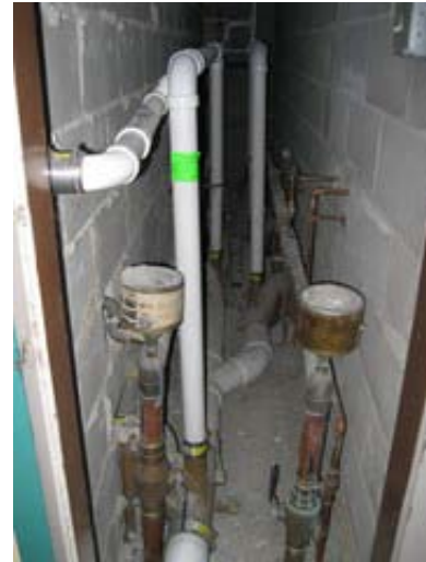
Sanitary Waste Lines
