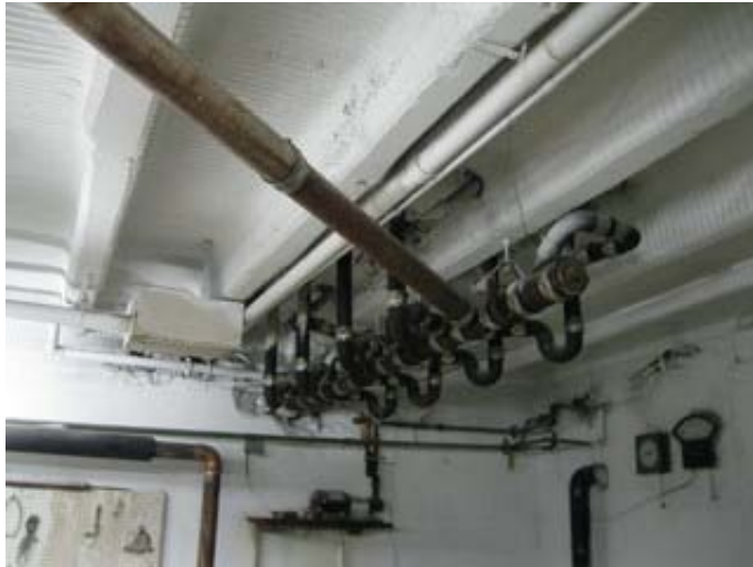
Sanitary Waste Lines
