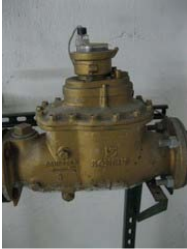
Incoming Domestic Water Service Meter
