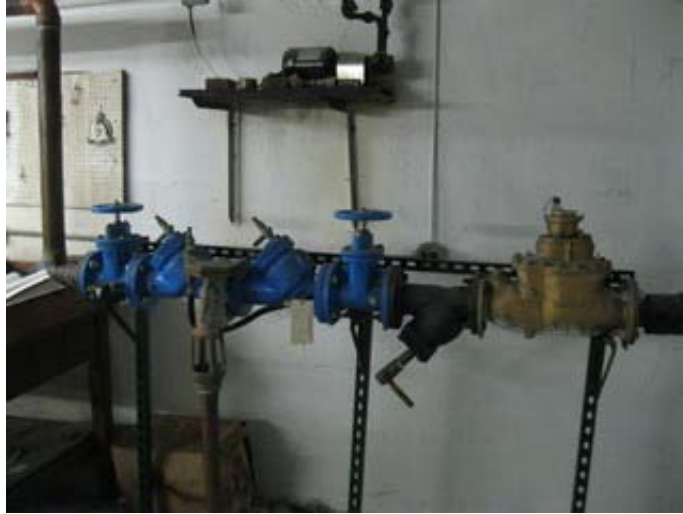
Incoming Domestic Water Service Line and Backflow Preventers
