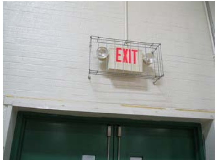
Non-Compliant Emergency Egress Light Fixture and Exit Sign
