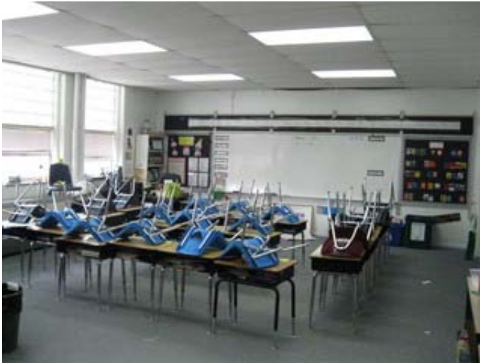
Classroom T-8 2x4 Lay-in Direct Fluorescent Light Fixtures
