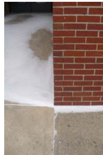
Minor Cracking in 1969 Addition
