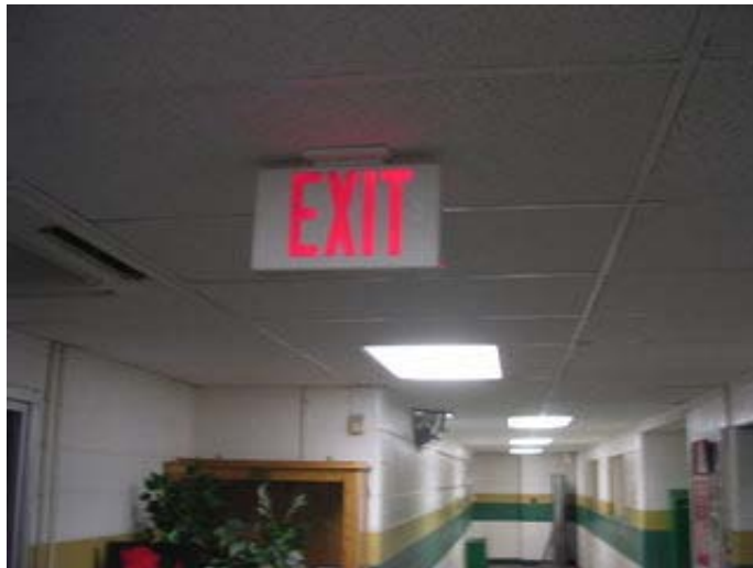
Typical Exit Lighting Signage
