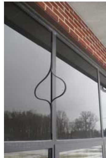
Poor Window Gasket in 1959 Addition
