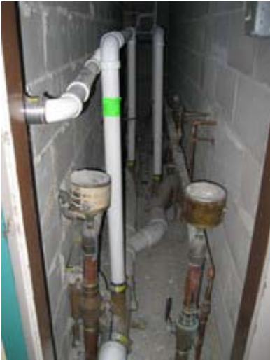
Sanitary Waste Lines
