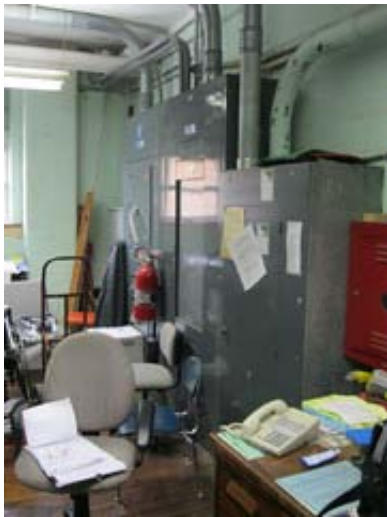
Main Electrical Distribution Panel
