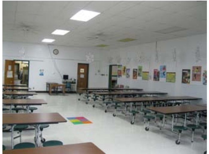
Student Dining T-8 2x4 Lay-in Direct Fluorescent Light Fixtures
