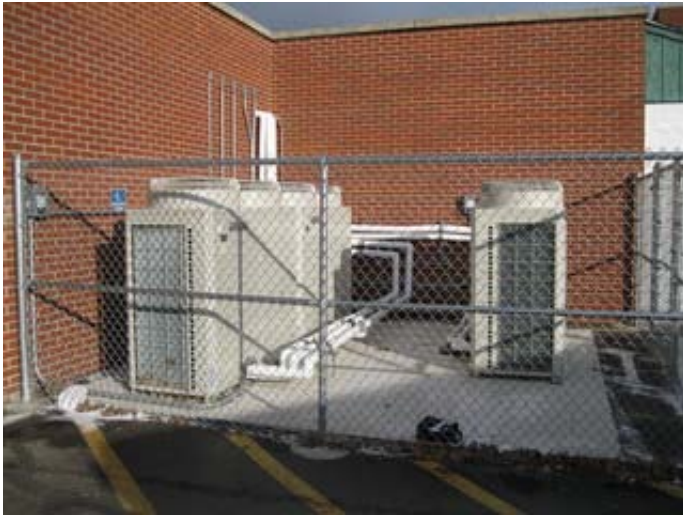
Mitsubishi Heat Pump Condensing Units
